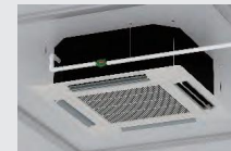
Installed in drainage pipe
